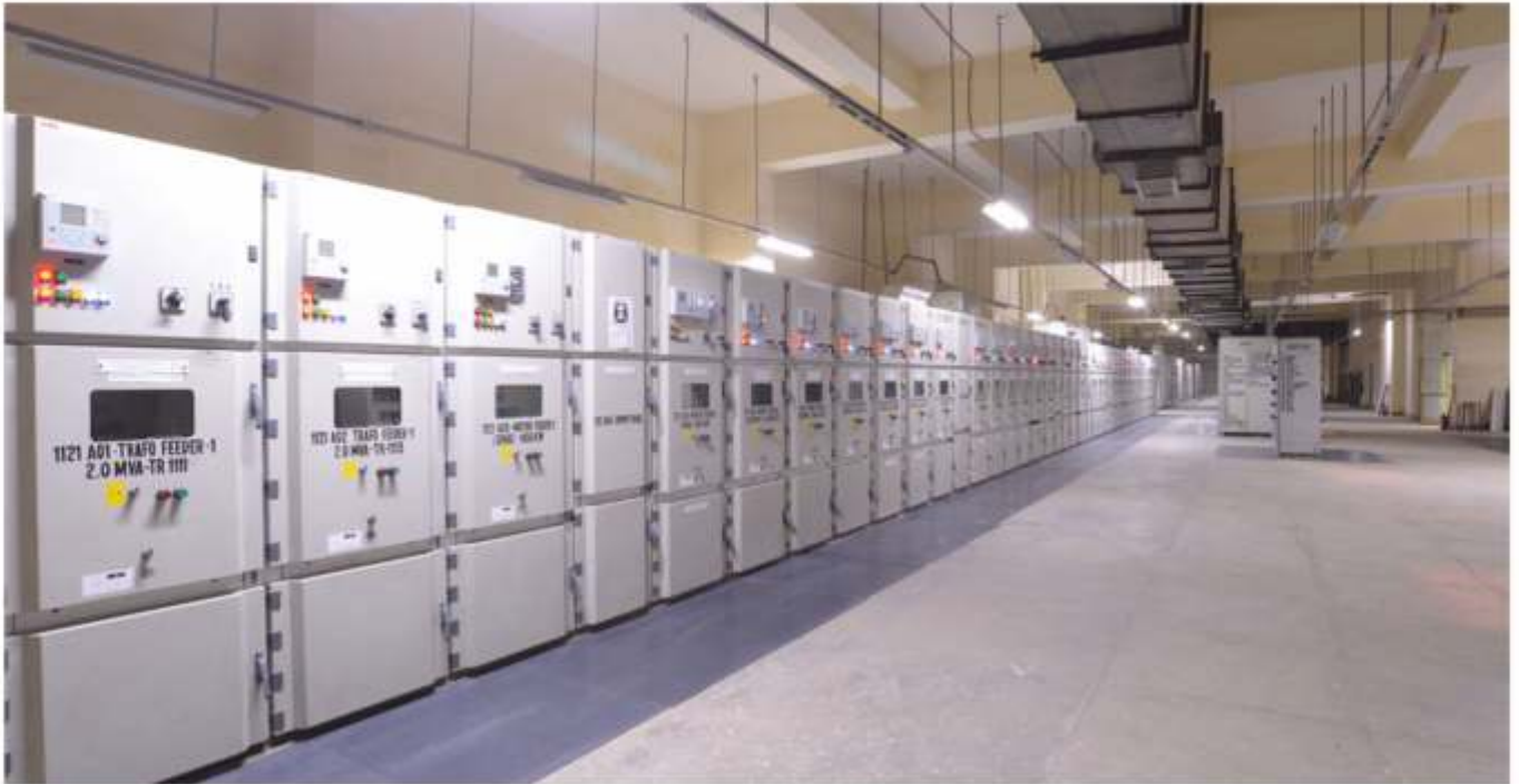
OPaL Plant's view at Dahej
