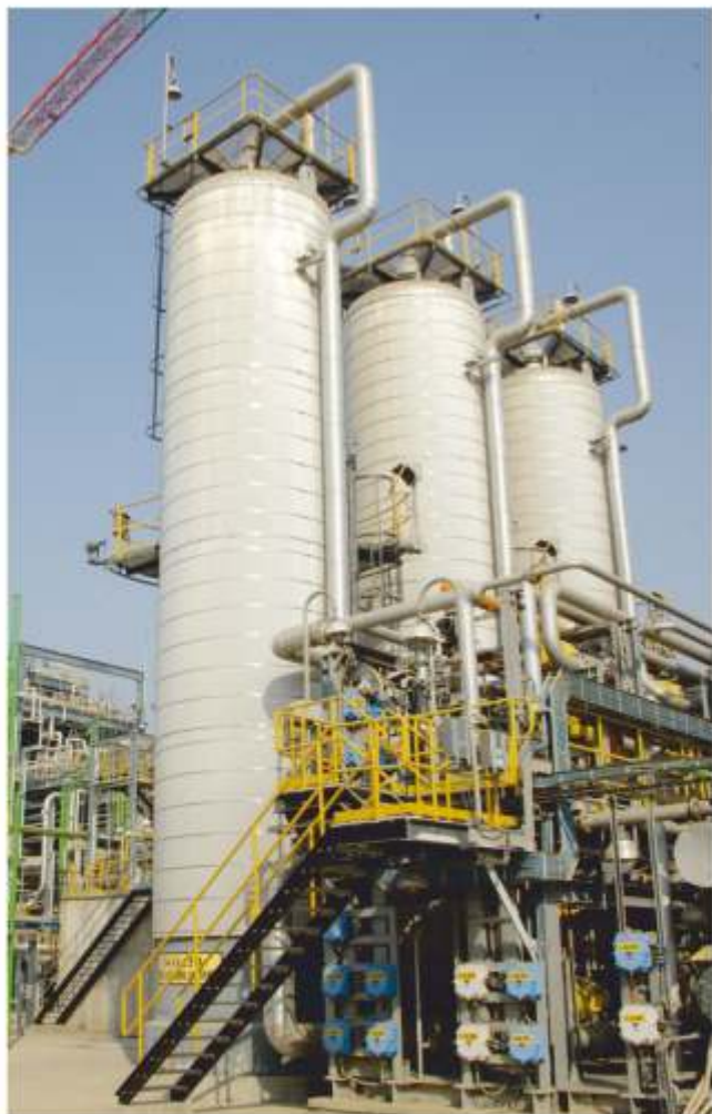
OPaL Plant's view at Dahej
