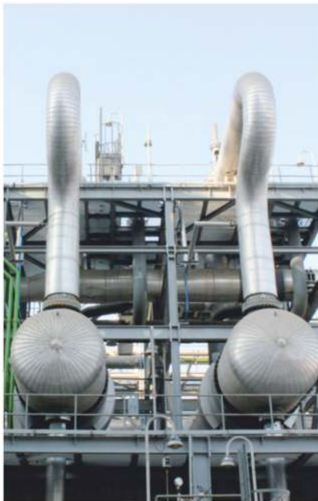
OPaL Plant's view at Dahej
